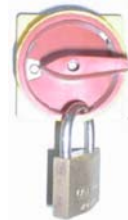
Main switch with padlock
